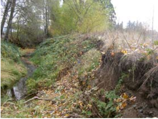
Figure 26.—Channel stability is important in site selection. Here, an overly steepened bank was cleared of dense blackberry cover, then planted. That winter, high stream flows washed away about 10 feet of bank along with most of the planted trees. Several years later, as seen here, parts of the bank were still eroding.
